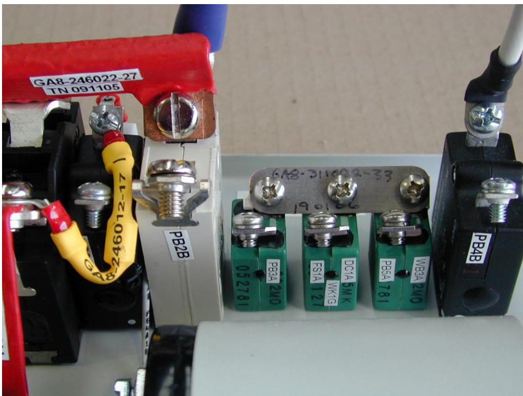
Figure 4 - Modified Breaker Assembly
